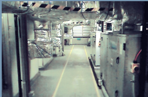
The DryCool™ system for the operating theaters was installed in the hospital's plant rooms.
